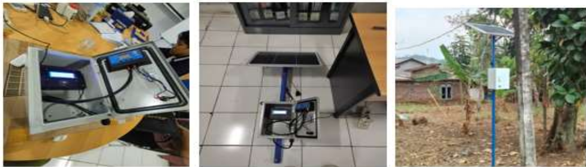
Fig. 4. Landslide early warning system
