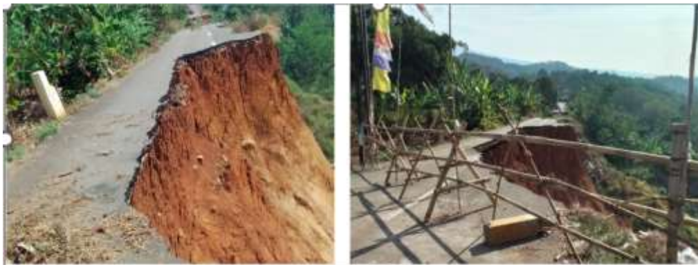
Fig. 2. Landslide conditions in Bandungan hamlet, Kalongan Village
