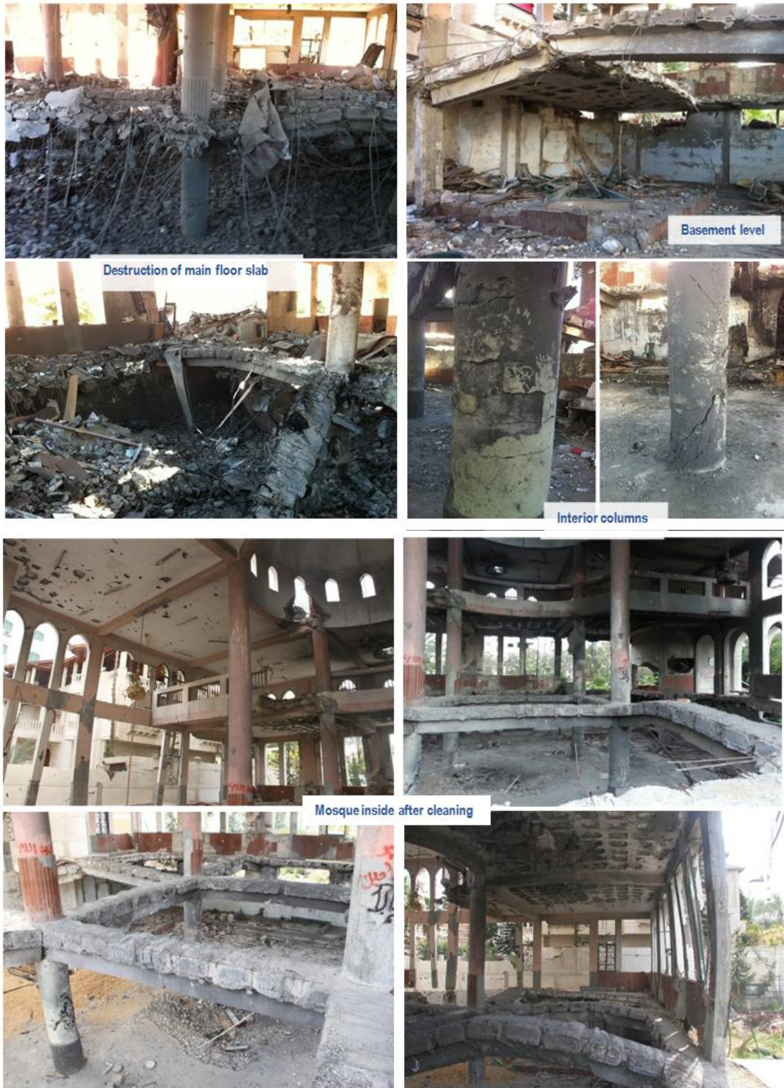
Fig. 3. Damage to Al-Amin Mosque- inside photos (before and after removal of debris)
